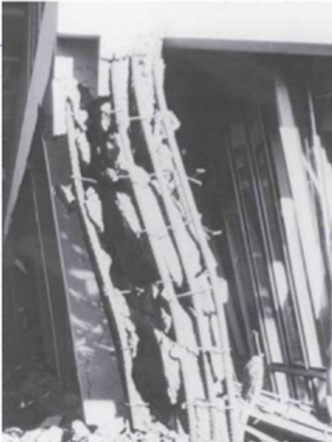
Tied col. destroyed in 1971 San Fernando earthquake
