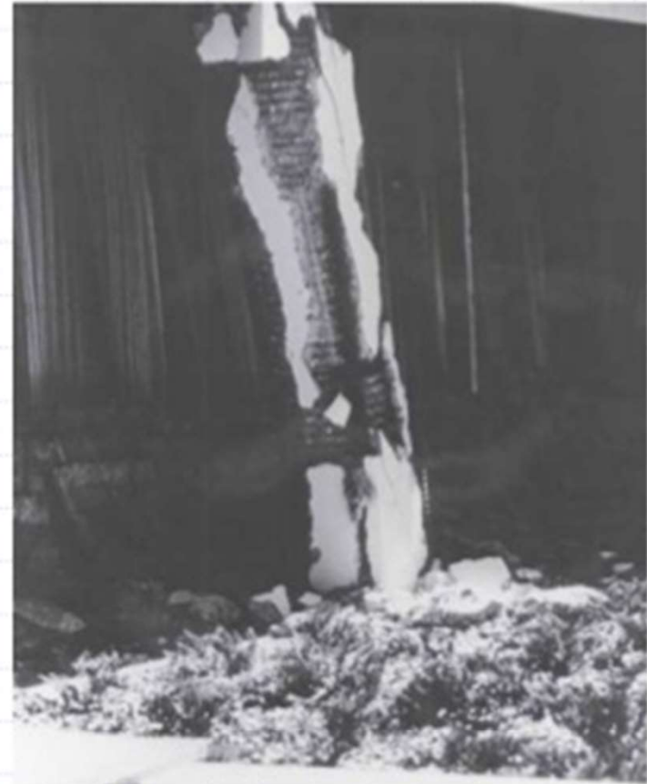
Although this column has been deflected sideways 50 cm, it is still carrying load
